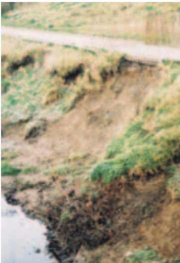
Failed riverbank before reconstruction
